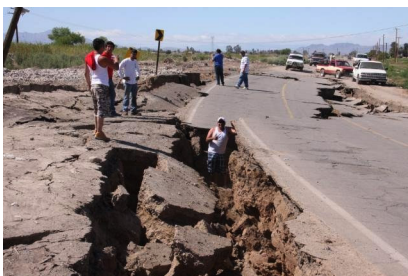
Street damage in Mexicali
