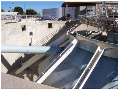
Damaged 10 M. Gallon clarifier
