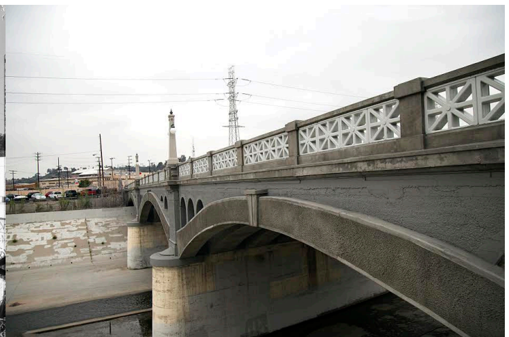
After: The project included restoration of the 1910 original design of criss cross railings and globe lights.
