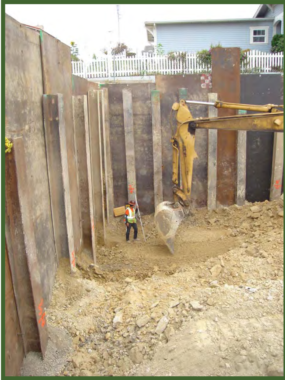
Pismo Heights-During Construction: Excavating down over 30 feet. The two-story house in the background, 30-feet above the floor level of the tank.
