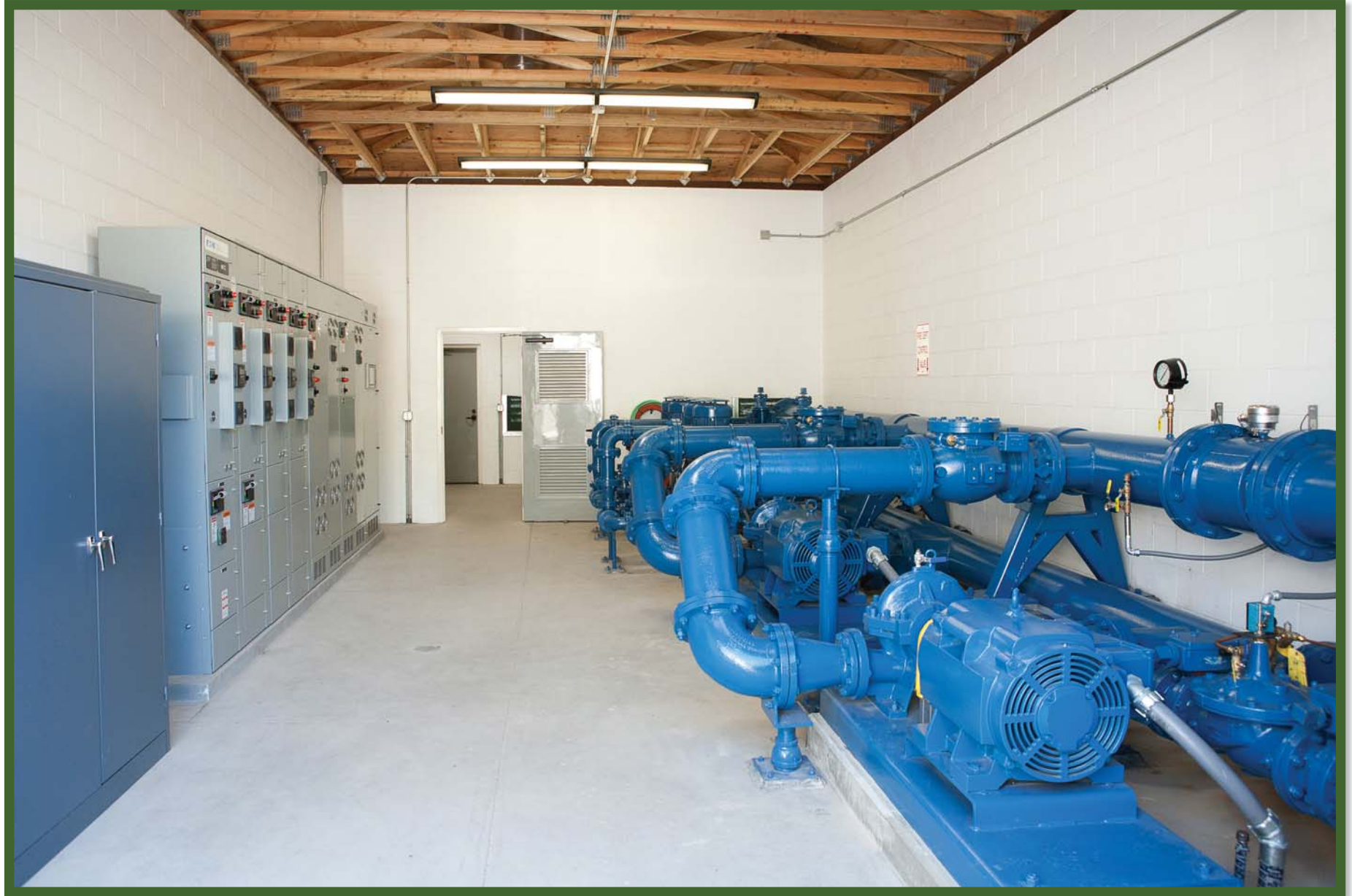
Pismo Heights-Main Control Room: The fire pump in the fore ground.
