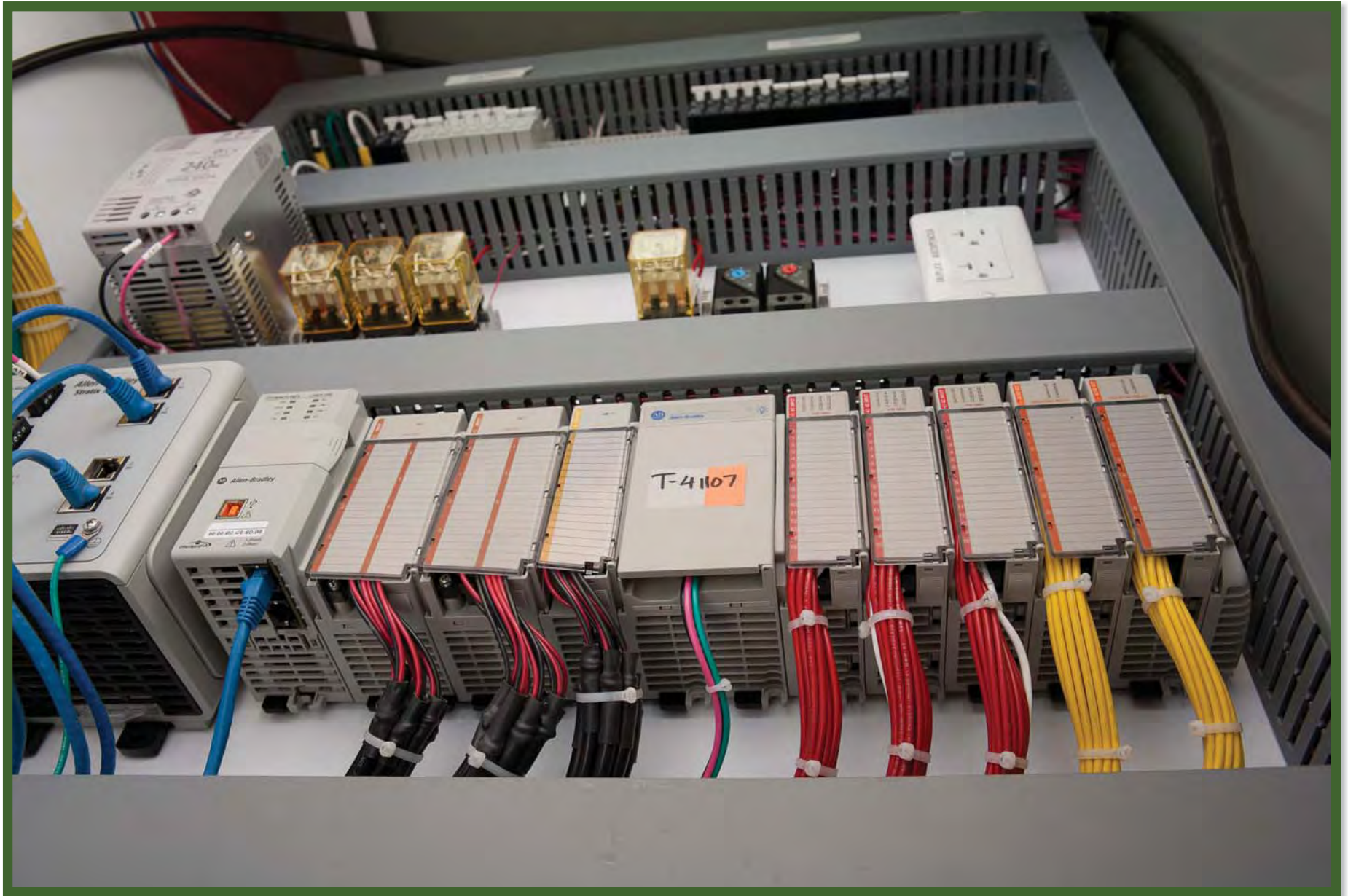
Pismo Heights-Main Control Room: The internal controls.
