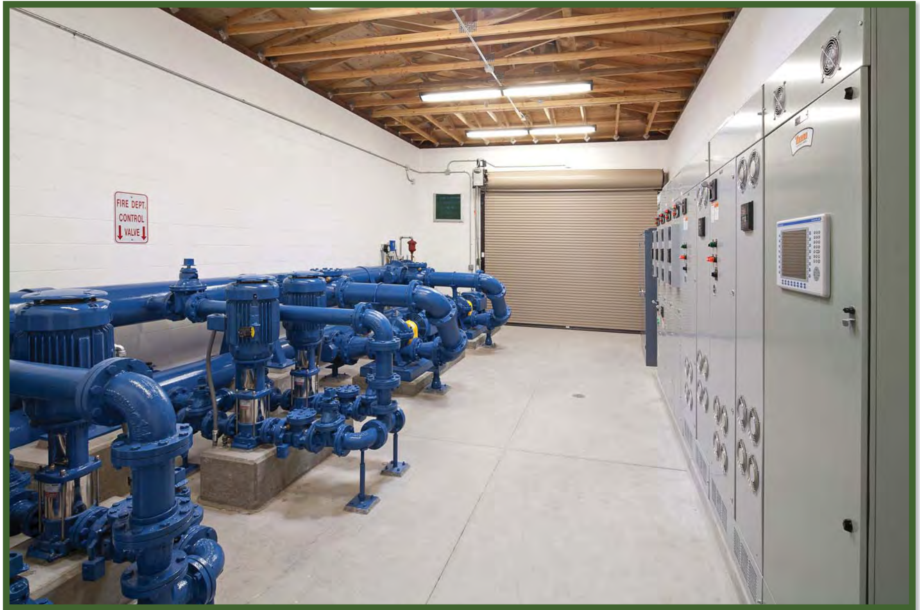
Pismo Heights-Main Control Room: The six pumps and control panels with the roll up door in the background.
