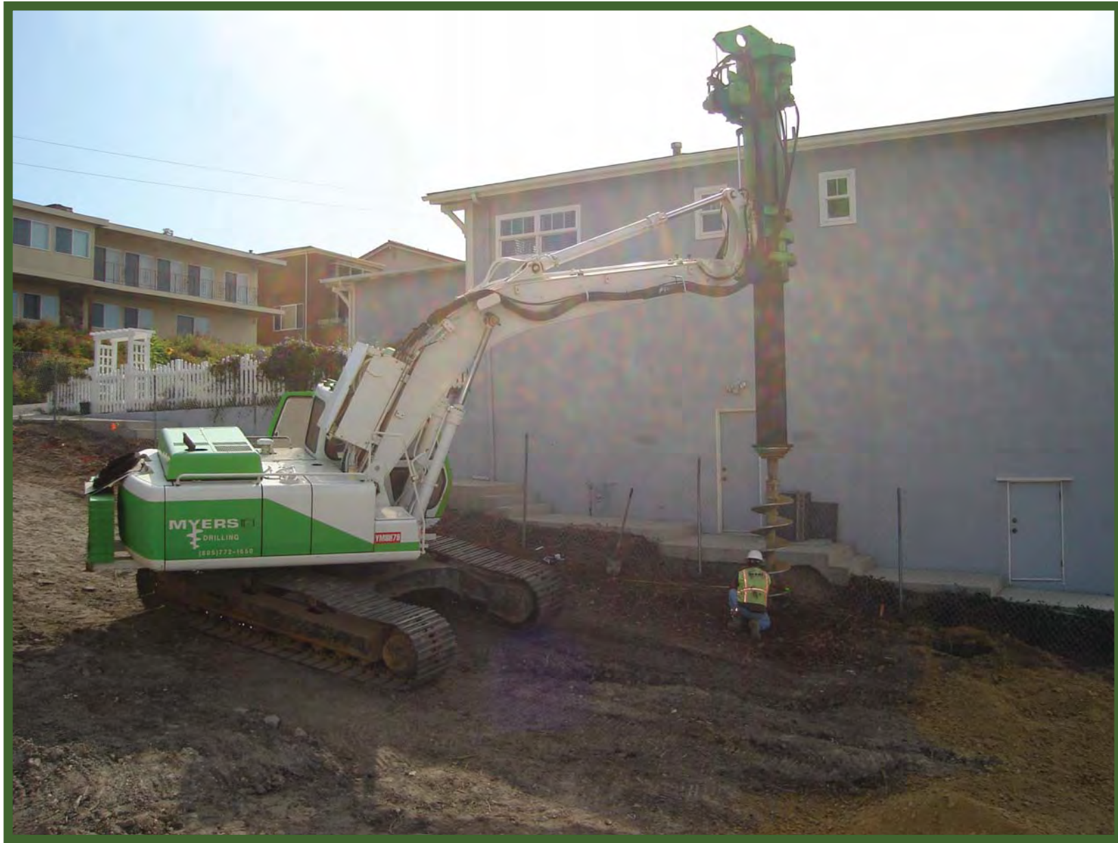
Pismo Heights-During Construction: Start of excavation for the tank. Drilling for install the pilings for the shoring. At ground level with the two-story house.
