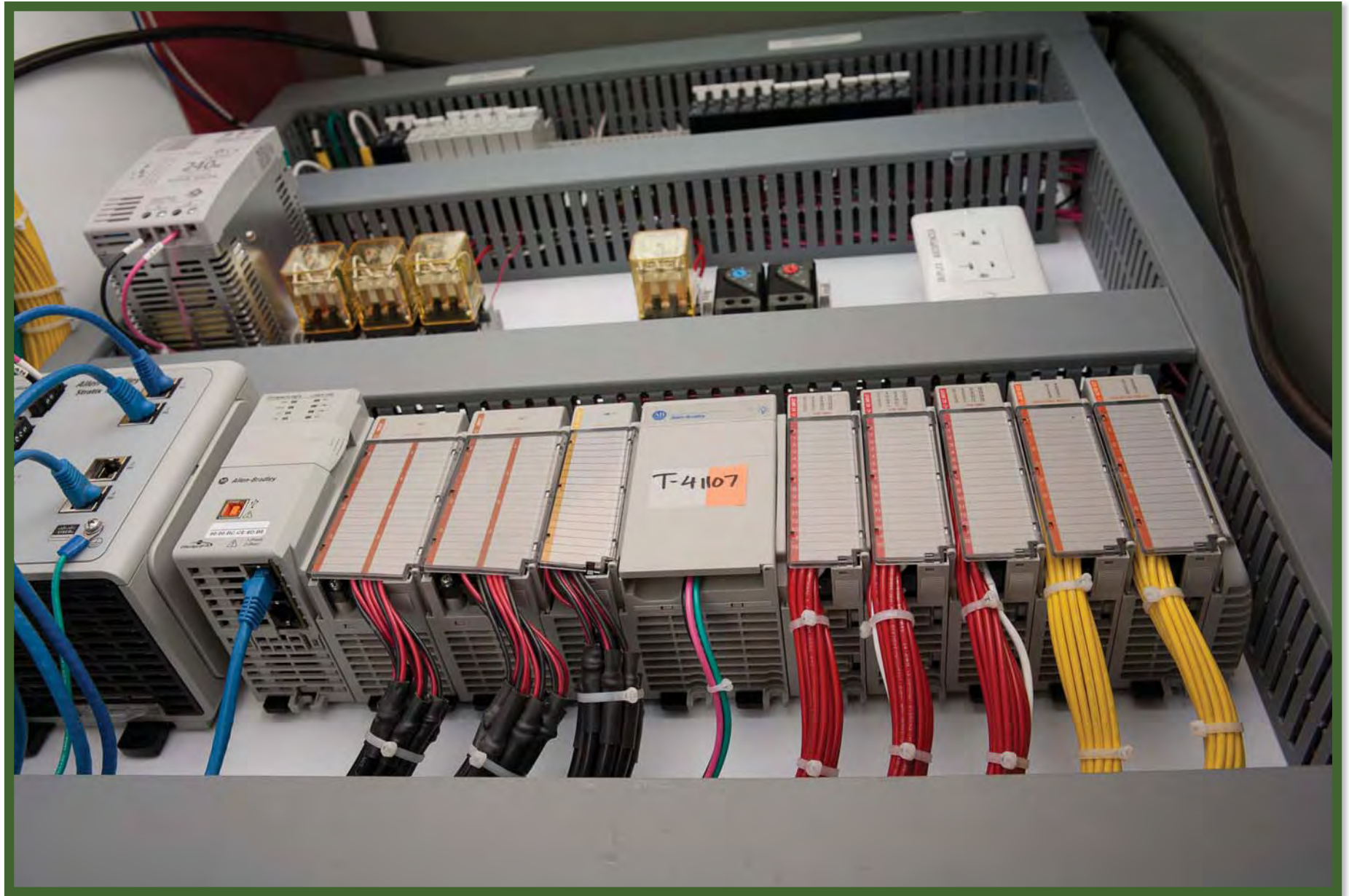
Pismo Heights-Main Control Room: The internal controls.
