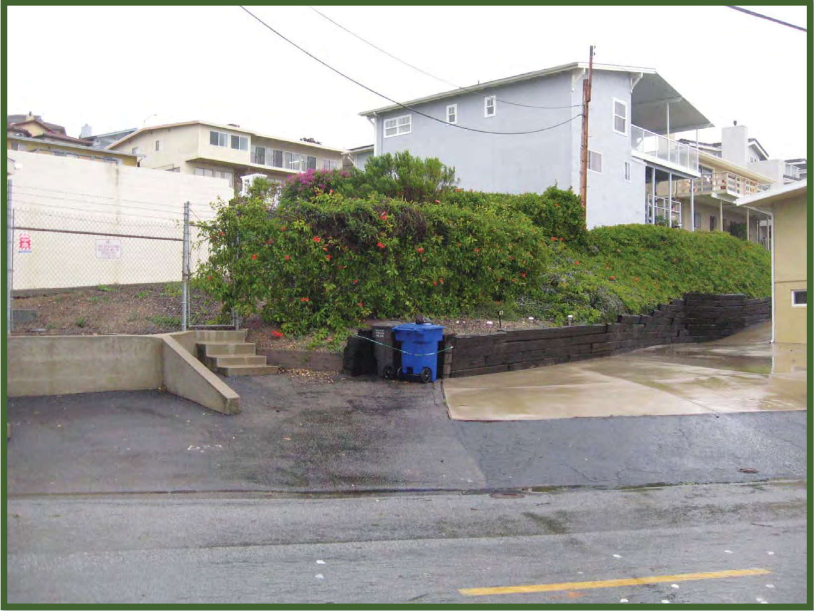
Pismo Heights-Before: Neighbor's driveway and failing railroad retaining wall.
