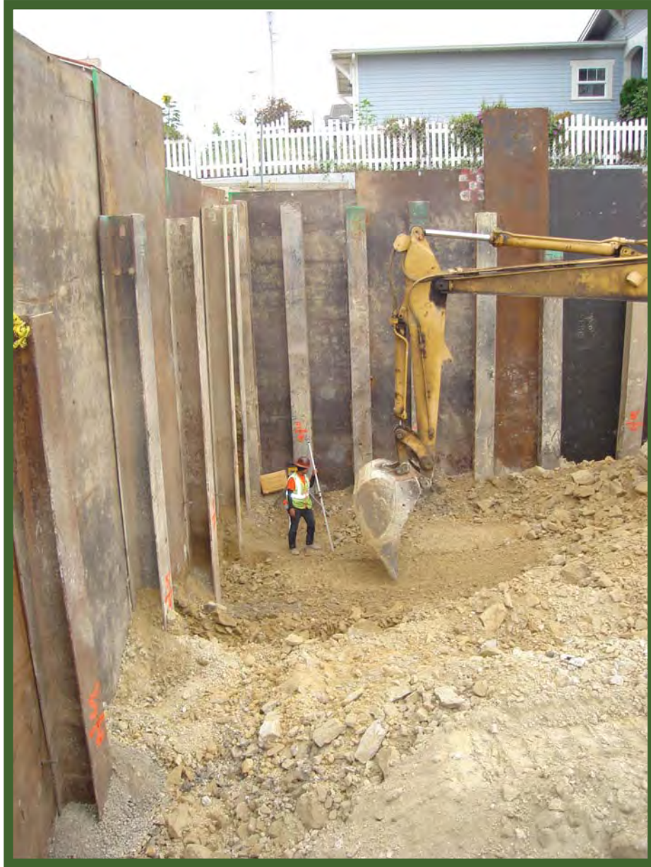
Pismo Heights-During Construction: Excavating down over 30 feet. The two-story house in the background, 30-feet above the foot level of the tank.
