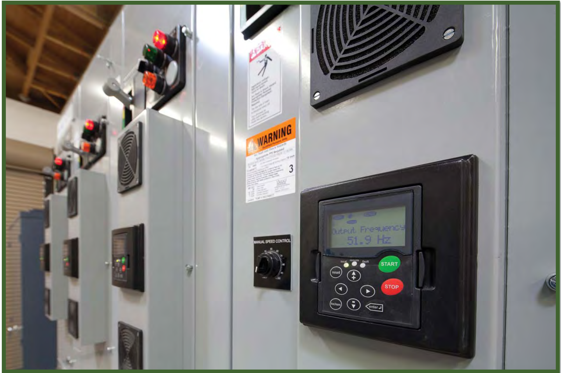
Pismo Heights-Main Control Room: The pump control panels.
