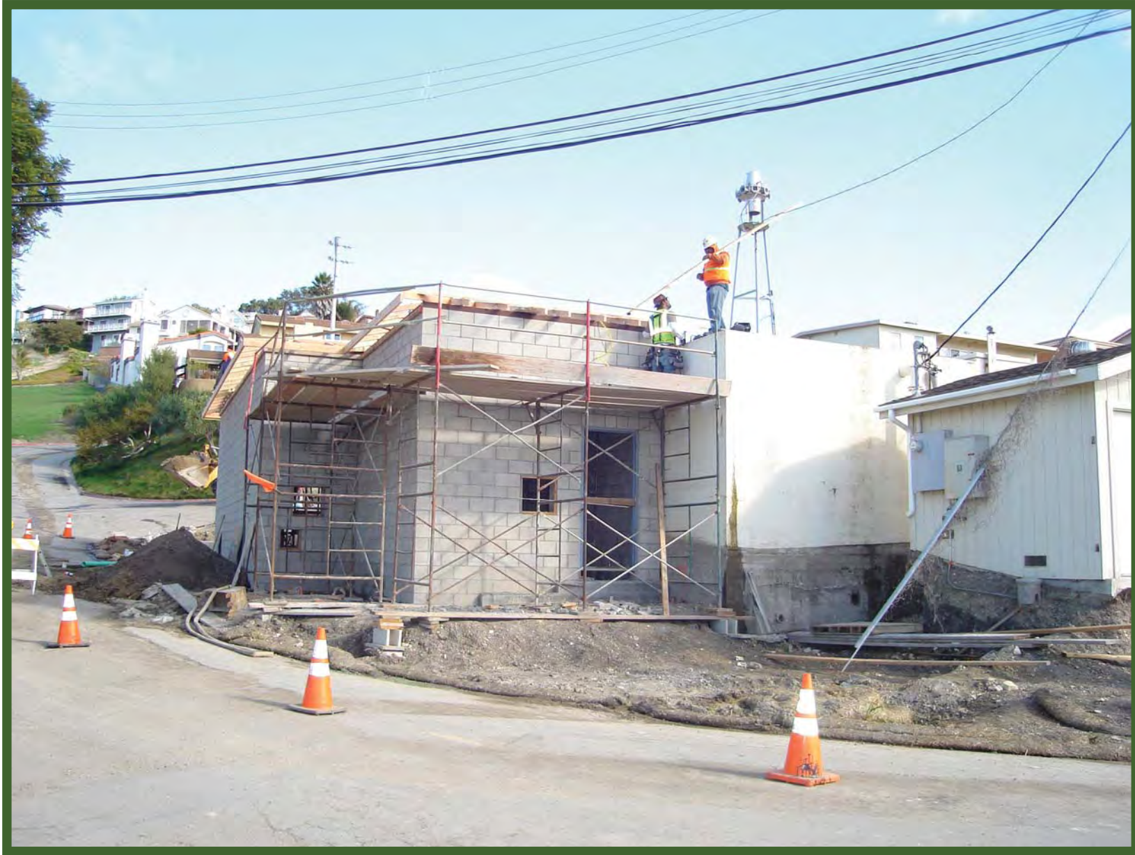
Pismo Heights-During Construction: Construction of the new booster station building. Note the existing booster station building still sitting on its foundation with the ground graded out around it.
