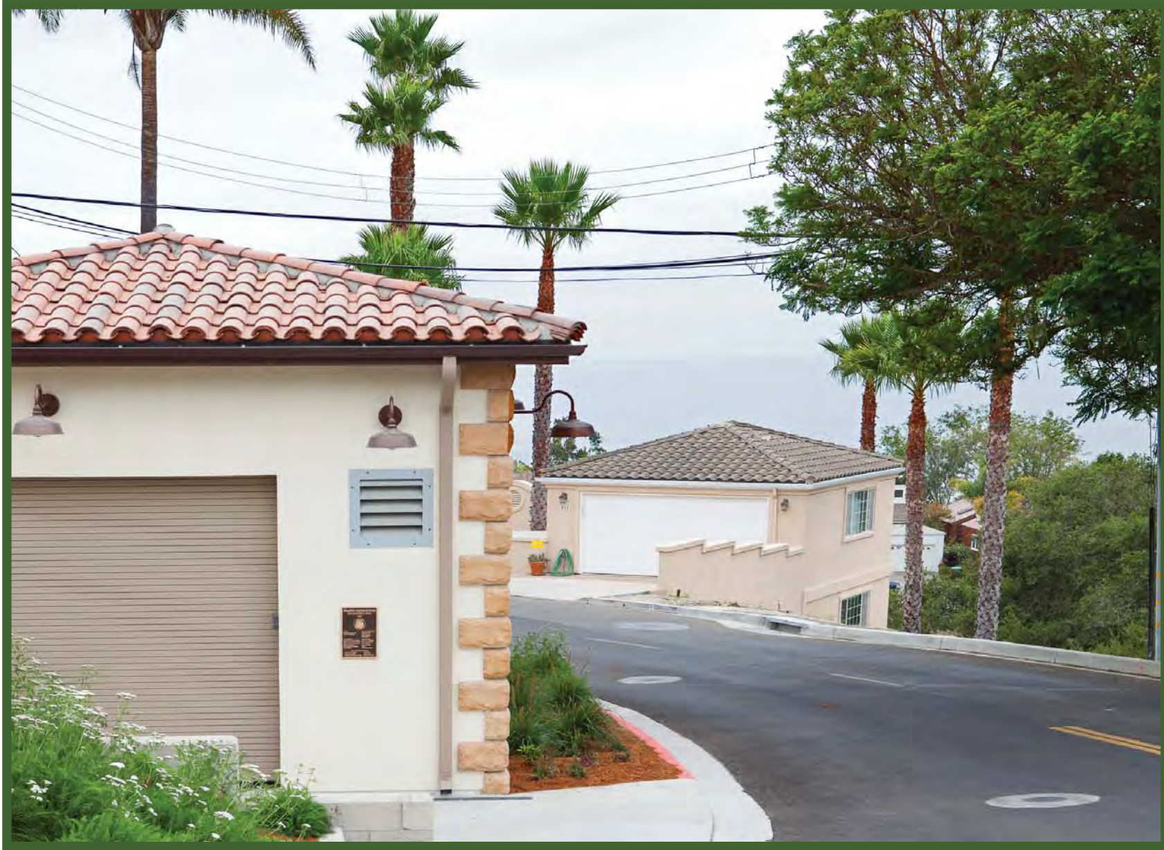
Pismo Heights-Finished Construction: Looking from the corner of Merced Street. The west portion of Longview Avenue on the right side of the picture was excavated down 9 feet and then re-compacted and then paved.
