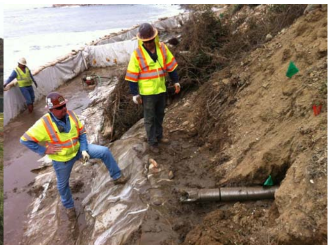
Dewatering Drain Breakout
