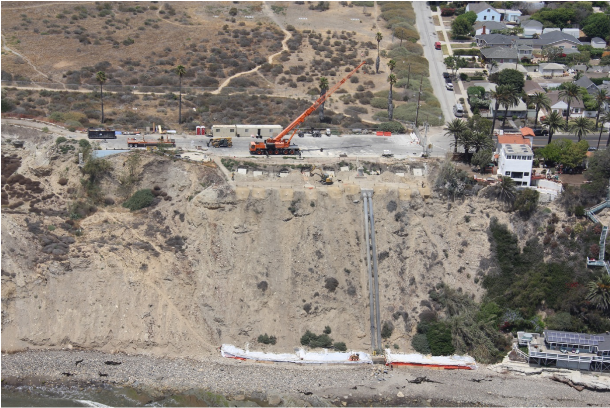
Completed Project – Dewatering entry pits (grey structures) at top of photo, dewatering drain outlets at base of bluff, and concrete anchor reaction pads in center of photo (pads are made of colored and textured shotcrete)
