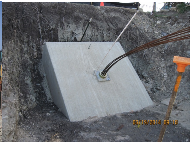
Concrete Anchor Reaction Pad
