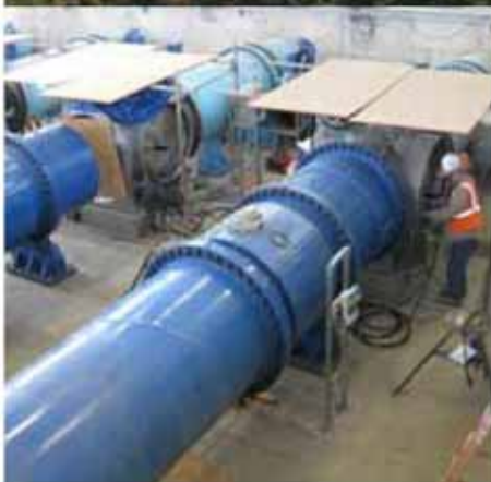
Los Angeles Aqueduct Filtration-UV Disinfection Plant: placing the field-fabricated 144-inch diameter inlet and outlet elbows to connect the plant with the water supply system. Insert: Reactor No. 1 being installed.
