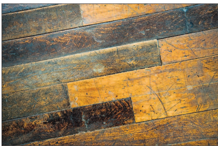
The original floors in the interior of the Packing House, made of maple planks, were preserved.
