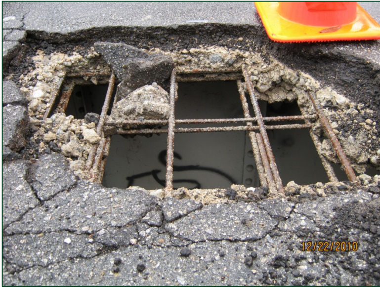
Rainstorms Washed Out Old Bridge Deck Exposing Reinforcement (December 2010)
